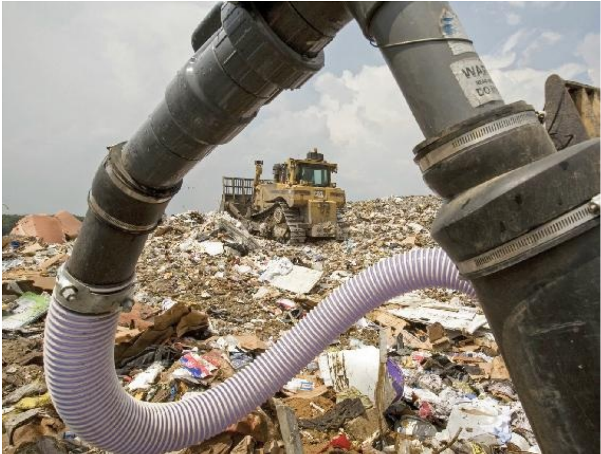
Wellhead for methane capture at a landfill in Michigan.
